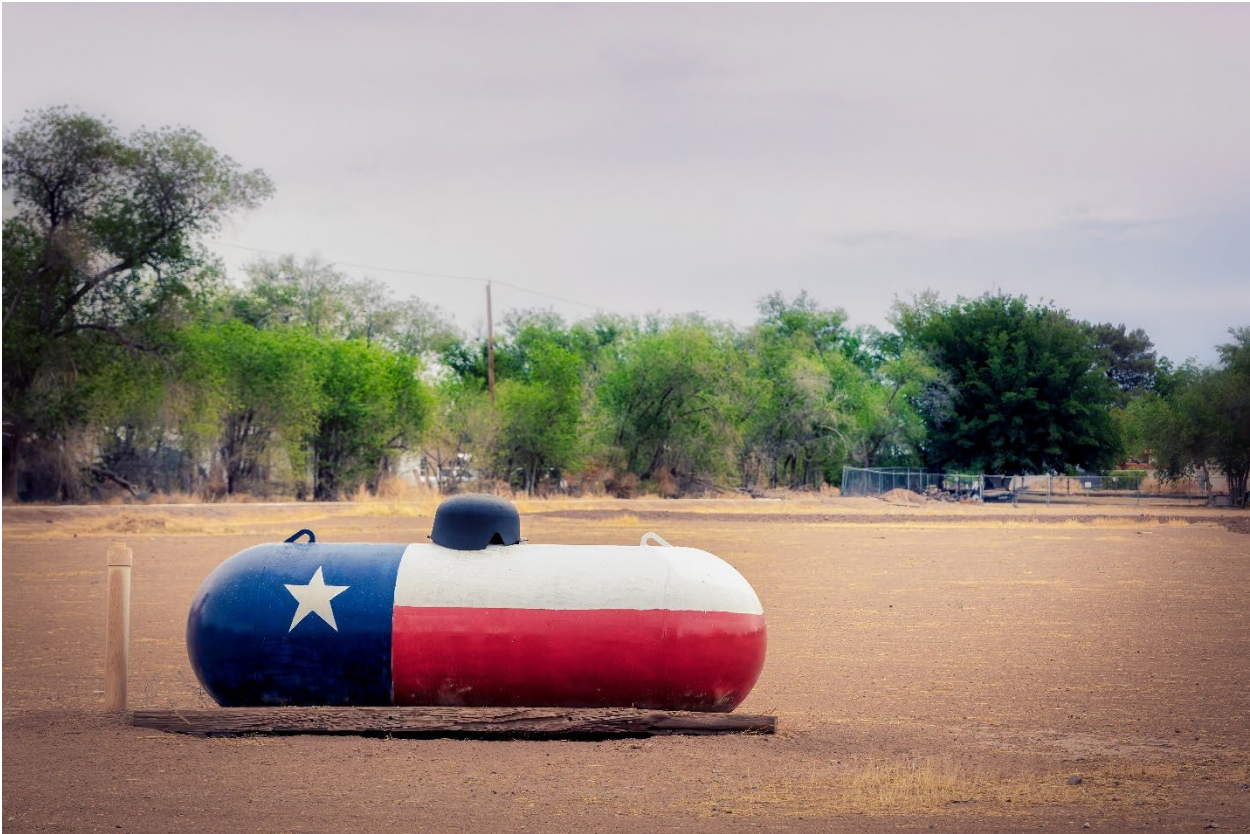
Figure 2-3. Propane Tank with Flag of Texas
